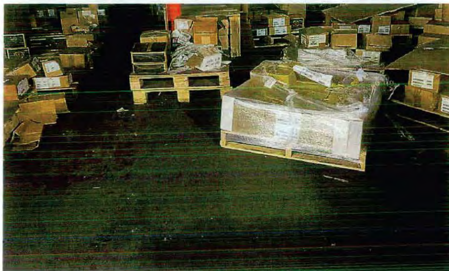
Photo 1: Interior Floor – view to the east of the northeastern portion of the building; visible portions of floor are in good condition with minimal shallow cracks.
