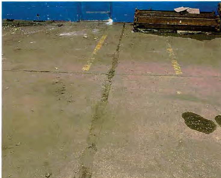
Photo 3: Interior Floor – view to the south of the floor in the southern portion of the building with a crack partially filled in.
